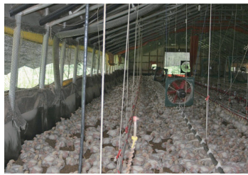
Lighting control chicken house
