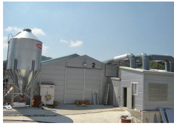
Geothermal heat pump system
