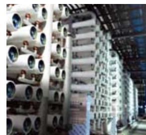
Hyundai Steel Industrial Water Channel
