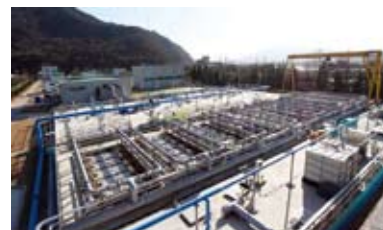
Daegu Dalseong Industrial Complex WWTP (25,000m 3 /day)
