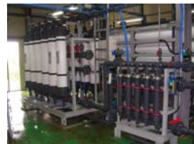
Seawater Desalination System
