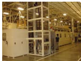
PowerTech America-Georgia Impregnation System
