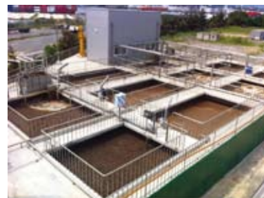
Ulsan Yongyeon Wastewater Treatment Plant Digestive Supernatant Treatment Facility
