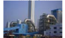
Dangjin Thermal Power Plant desulfurization facility
