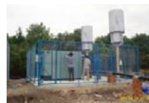
Started operating incinerating landfill gas (June 2010)
