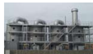
SK Innovation NMP Recovery Facility
