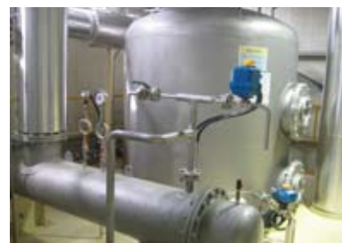
Donghee Auto Wastewater Zero Discharge Site
