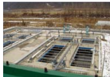
Daedeok Industrial Complex Phosphorous Treatment Site
