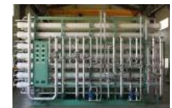
Mexico R/O Facility
