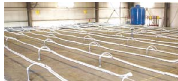
Dynamic electricity purification
