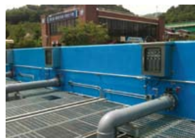
Gyeonggi Gapyeong Sewage Treatment Plant, Advanced Sewage Treatment (Total Phosphorous Treatment)
