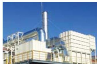
GM Korea-Changwon Plant Advanced RTO System
