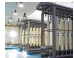
Yeongdeungpo Arisu Water Purification Center (Pressurized, 25,000t/d)
