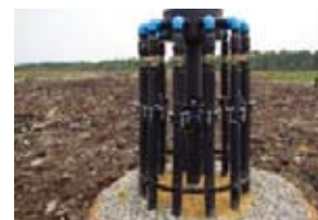
Landfill gas collecting facility (Dec 2010)
