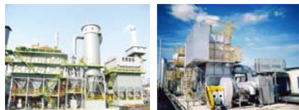
Combustion gas treatment system
