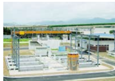
Jangnim Wastewater Treatment Plant
