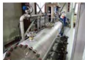
Sewage sludge reduction facility
