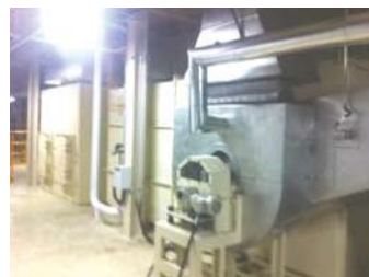
GM Korea-Gunsan Plant Green Dry Oven System
