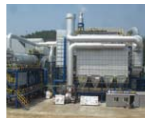
TKP Pohang oil reservoir worksite
