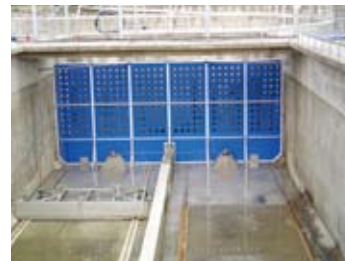
Gangbuk Water Purification Site
