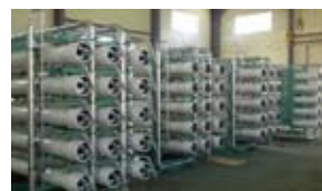
POSCO Mexico Plant, R/O System
