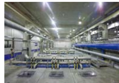
Yongin Sewage Treatment Plant
