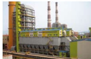
POSCO Gwangyang Iron Co, 5 sintering exhaust purification facility
